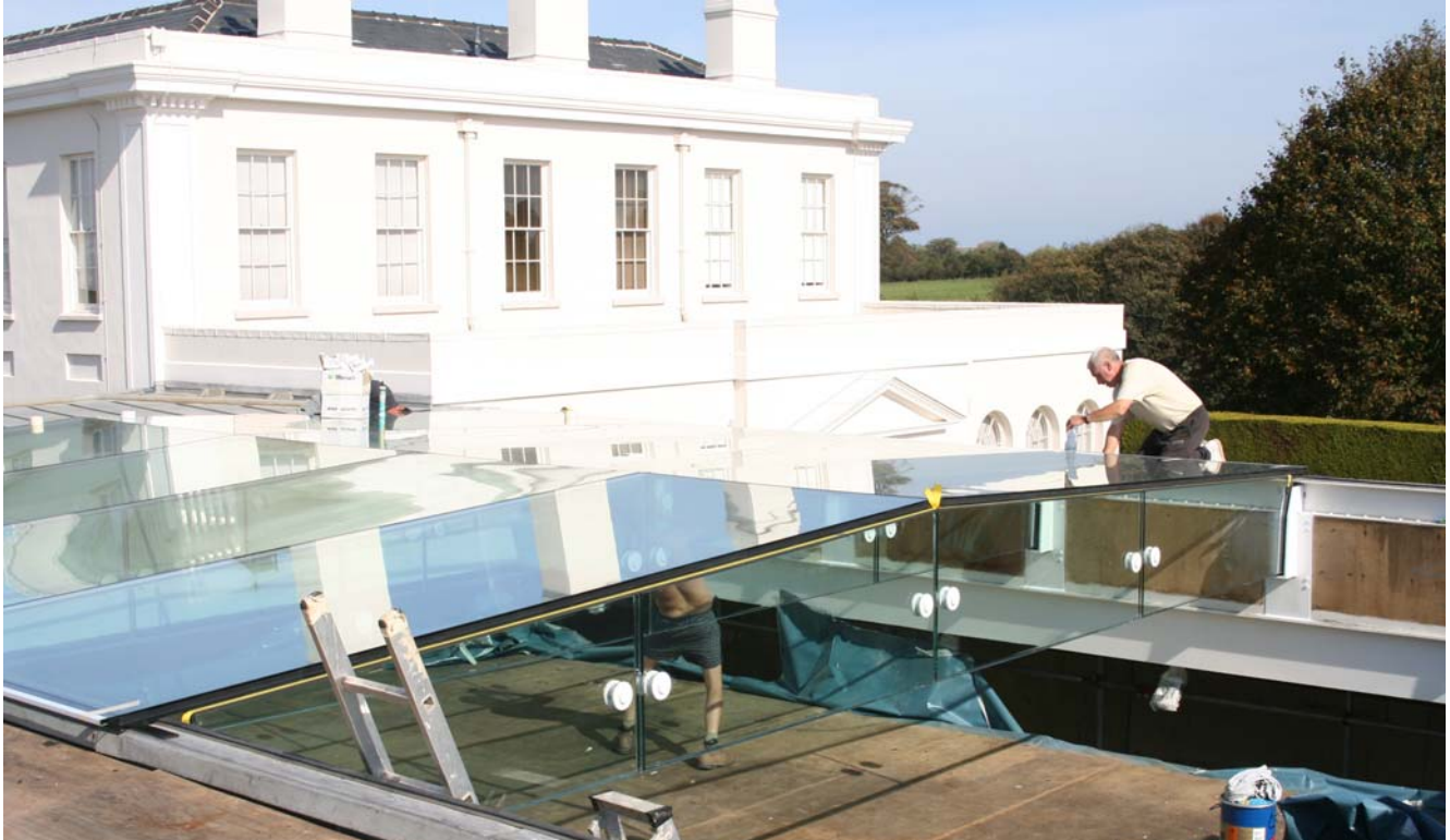
Low maintenance glass beams support the new roof over the swimming pool on a private estate in Guernsey - the first time structural glass has been used in this way on the island. (For further details, see Page 2, column 1)
