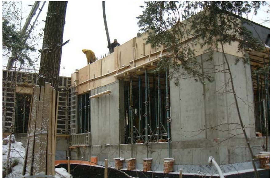
High quality finishes have been achieved on the concrete surfaces of the main building
